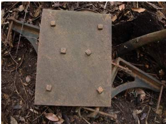
Figure 4.14 Head plate with dislodged angle brackets. (Photo: P1070066)
