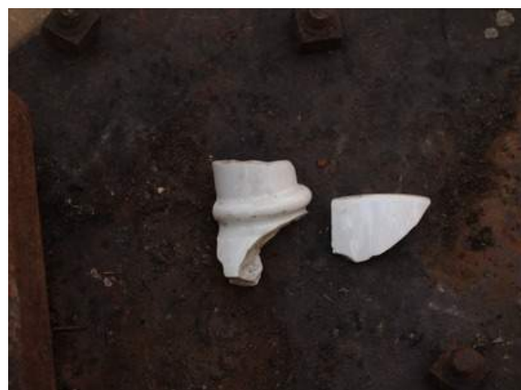
Figure 4.27 Fragments from a porcelain insulator used on telegraph tower. (Photo: P1020083)
