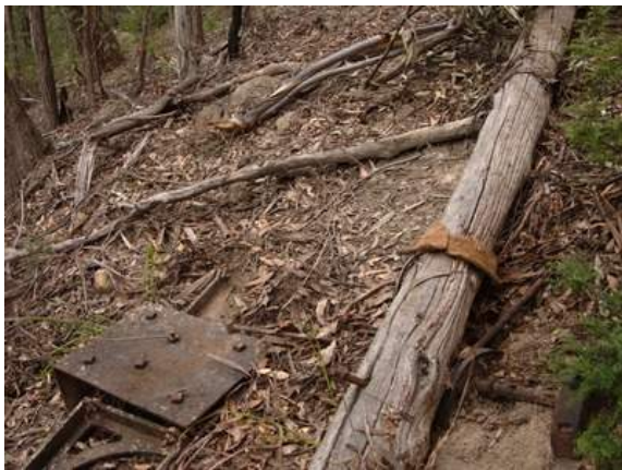
Figure 4.12 Fallen tower pole with headplate and bracket nearby. (Photo: P1020500)
